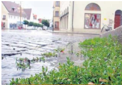
Problem: Clogged drains
